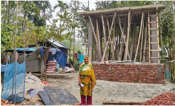
RHL project beneficiary in front her under construction resilient house. Photo: GJUS
